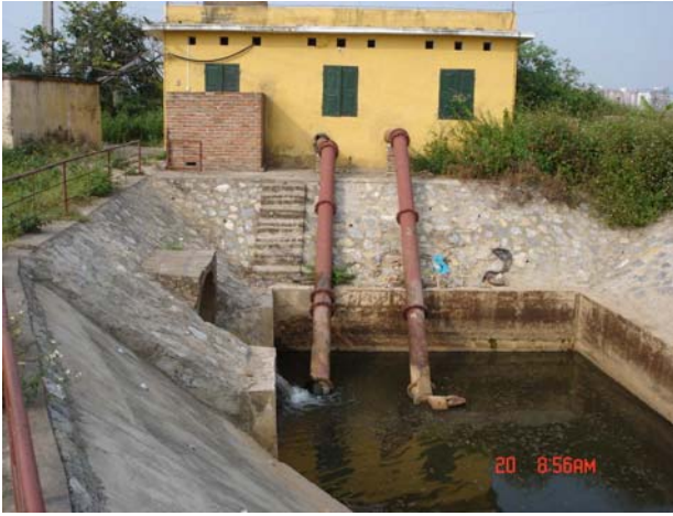
Figure 2 Waste water pumping station Bang B village
